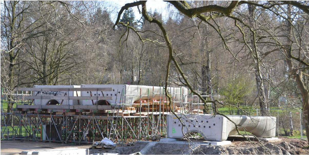
Figure 3.23: Assembly of individual girders on temporary formwork and loading to ULS, courtesy of De Gelderlander (Paul Rapp)
