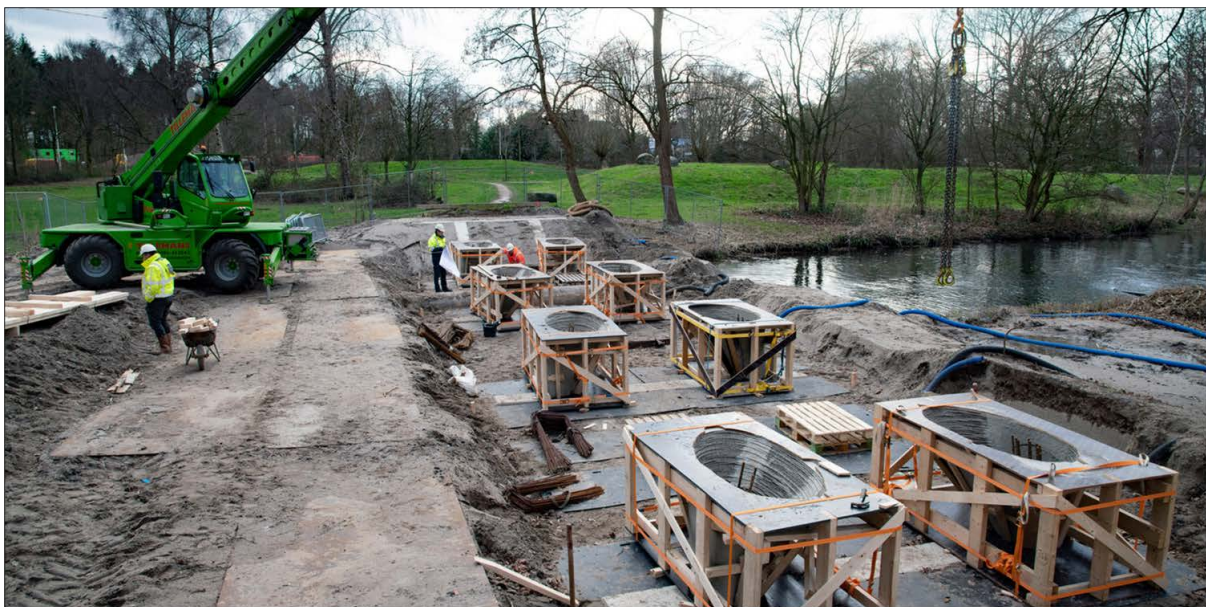
Figure 3.24: Assembly of printed formwork for bridge columns, with temporary supports, just before casting, courtesy of De Gelderlander (Paul Rapp)
