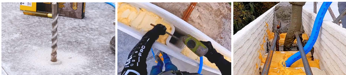
Figure 4.3: From left to right: drilling a hole for chemical anchoring of the rebar; inserting the rebar into the cavity after the structure has been printed; and subsequently casting or grouting the reinforcement to anchor it to the floor. Images taken from a video from Apis Cor homepage [82].
