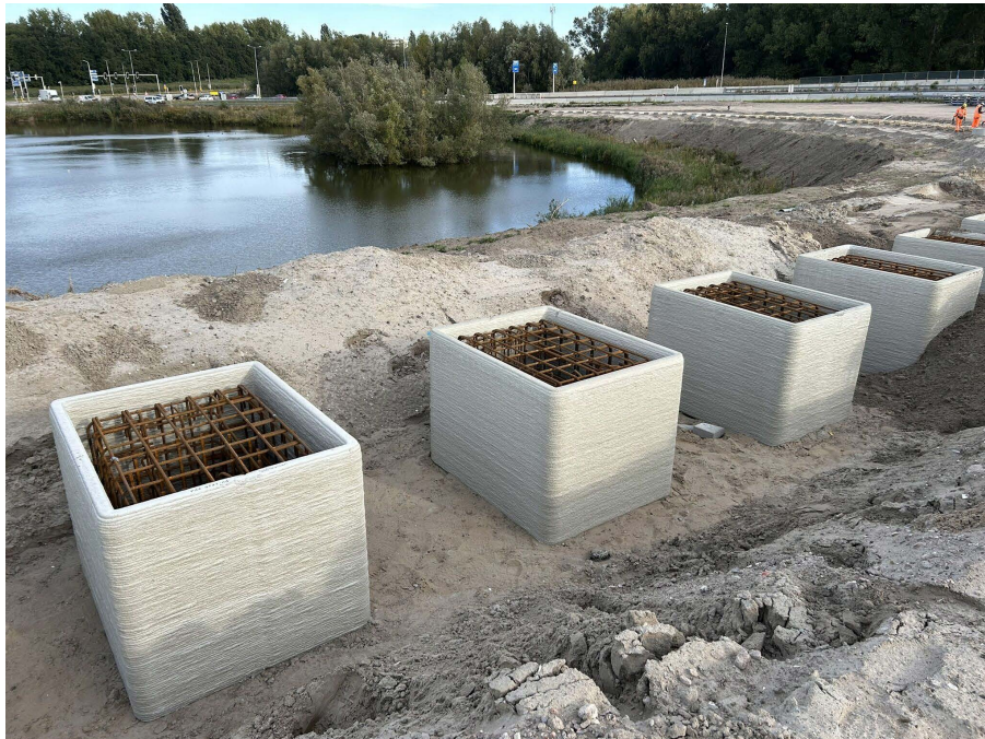
Figure 5.13: 145 pieces of printed formwork by Saint Gobain Weber Beamix, for the widening of A9 highway. The blocks are the foundation for a noise barrier wall. Taken from [54].
