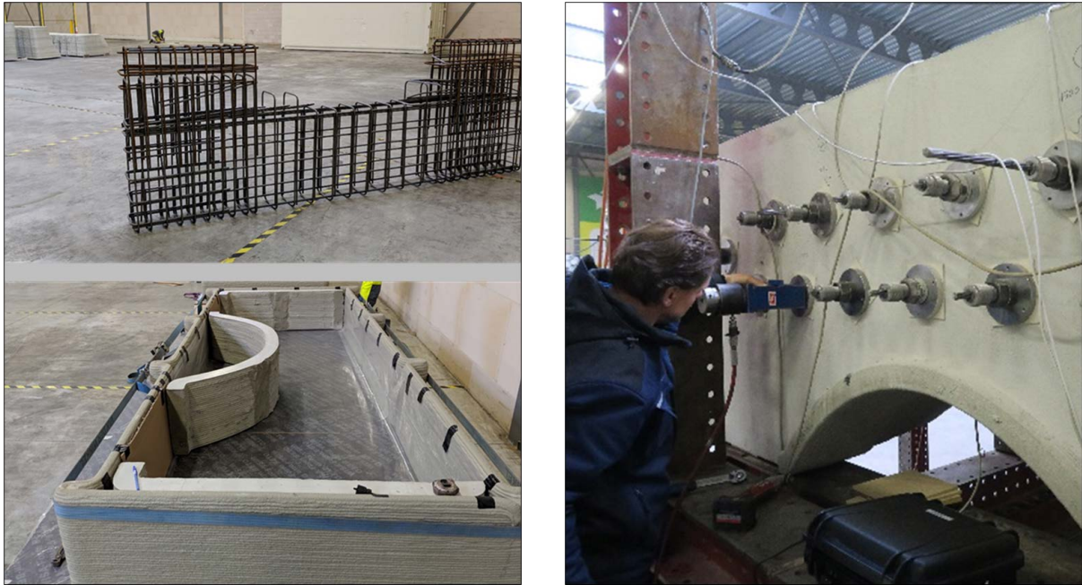
Figure 5.22: Reinforced anchor blocks were cast in 3D-printed formwork, and post-tensioning of tendons.
