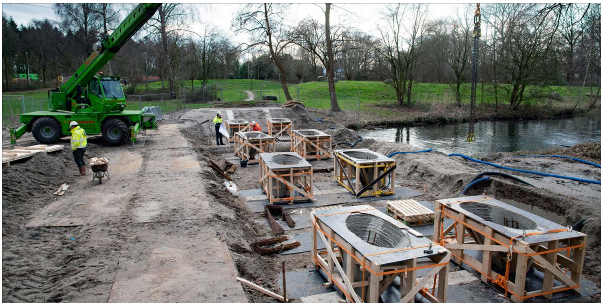
Figure 5.23: Assembly of printed formwork for bridge columns, with temporary supports, just before casting, courtesy De Gelderlander (Paul Rapp).
