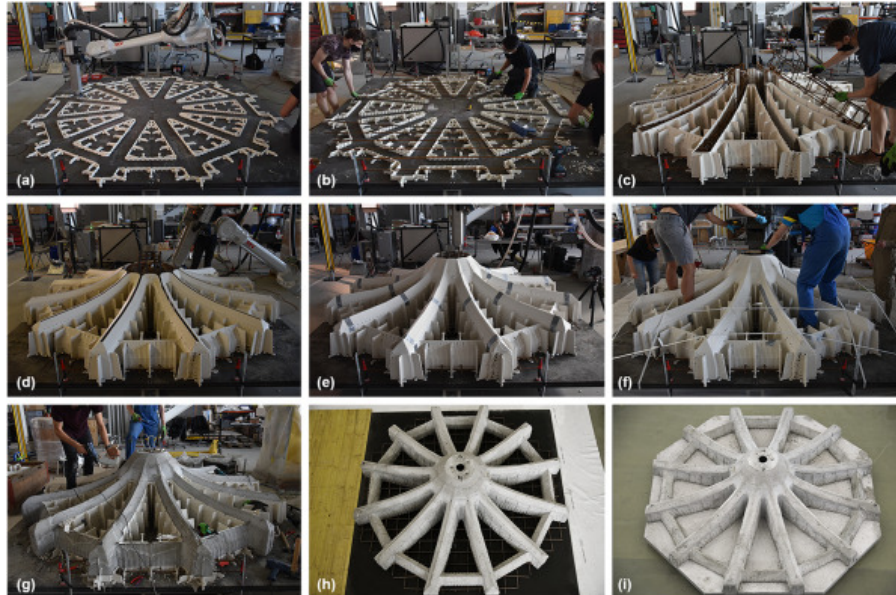
Figure 5.33: “Fabrication steps of the prototype. (a) 3D Printing bottom 35 mm, (b) placing slab reinforcement, (c) placing rib reinforcement cages, (d) 3D printing cap formwork, (e) 3D printing column-slab transition, (f) casting of rib formwork, (g) demoulding of ribs, (h) cast and demoulded ribs, (i) complete slab prototype after casting of the solid part of the slab” [62]. Taken from [62]
