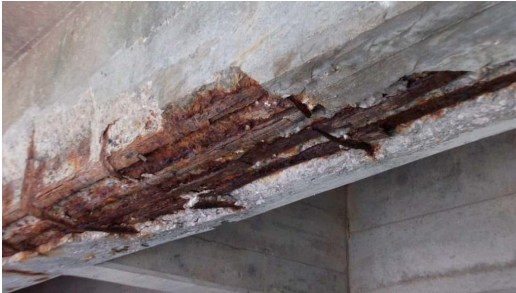
Figure 2.11: Example of durability-related deterioration in reinforced concrete: corrosion of reinforcement leading to cracking and spalling of the concrete cover (taken from Figure 1 in [11]).
