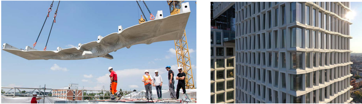
Figure 2.15: Left: Smart Slab in the Dfab House. Right: Domino Sugar site A.
